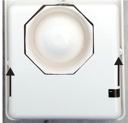
Photo 2 Internal protective cover of the siren
